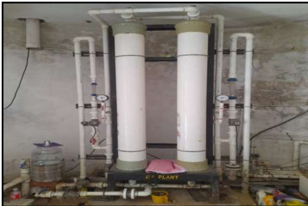
Ultra Filtration Plant
