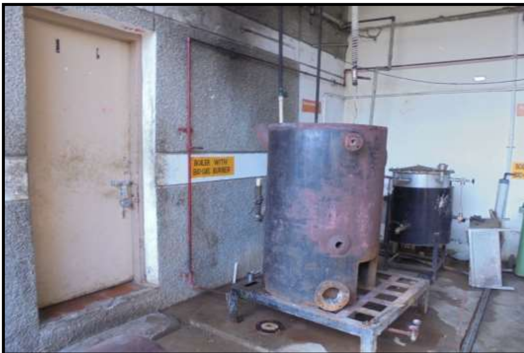
Boiler with Bio-Gas Burner
