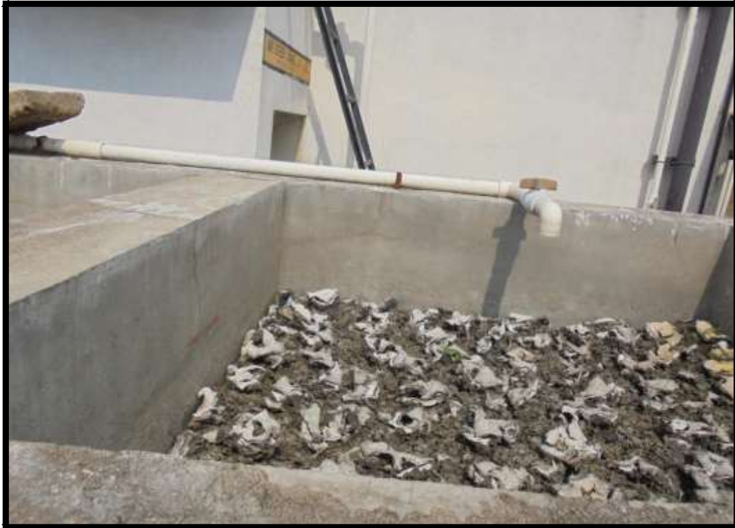
Sludge Drying Bed
