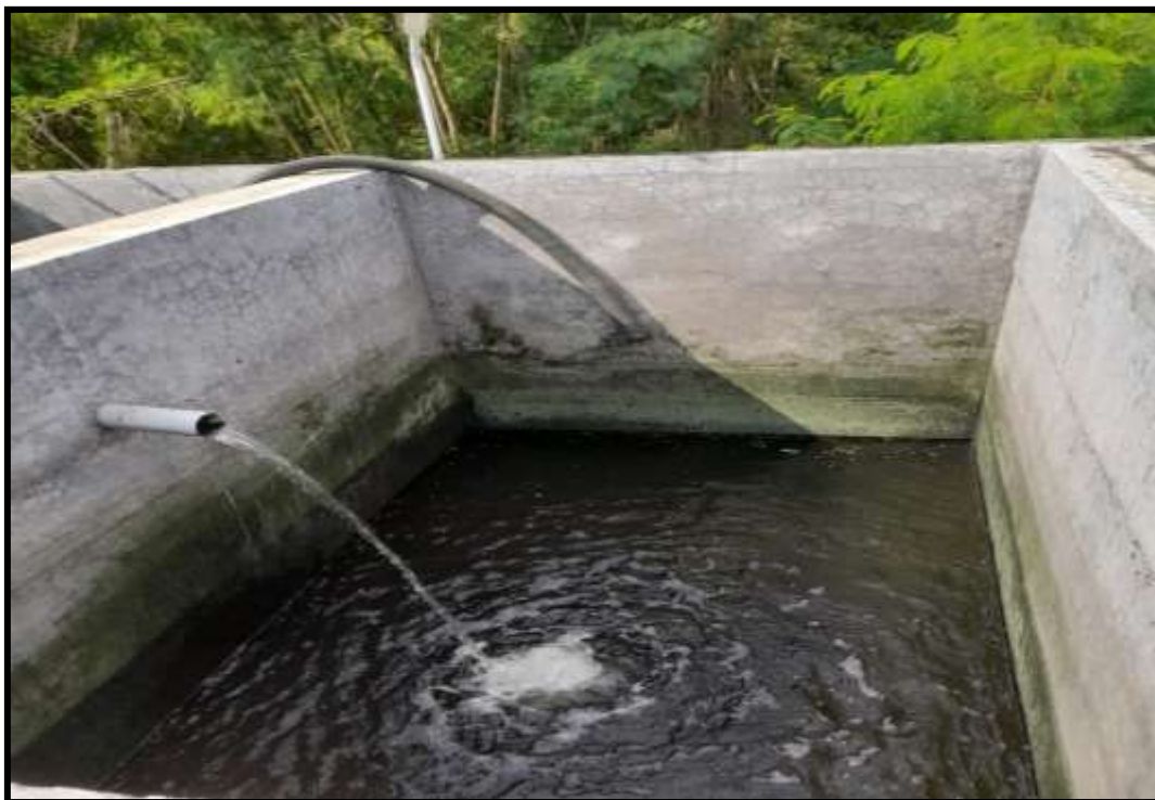
Clarified Water Storage Tank
