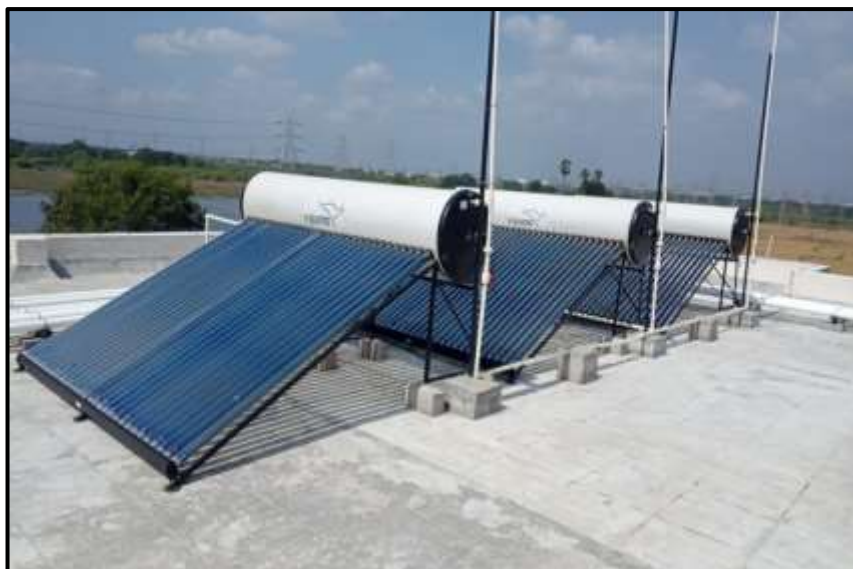
Solar Geysers installed above Hostel blocks
