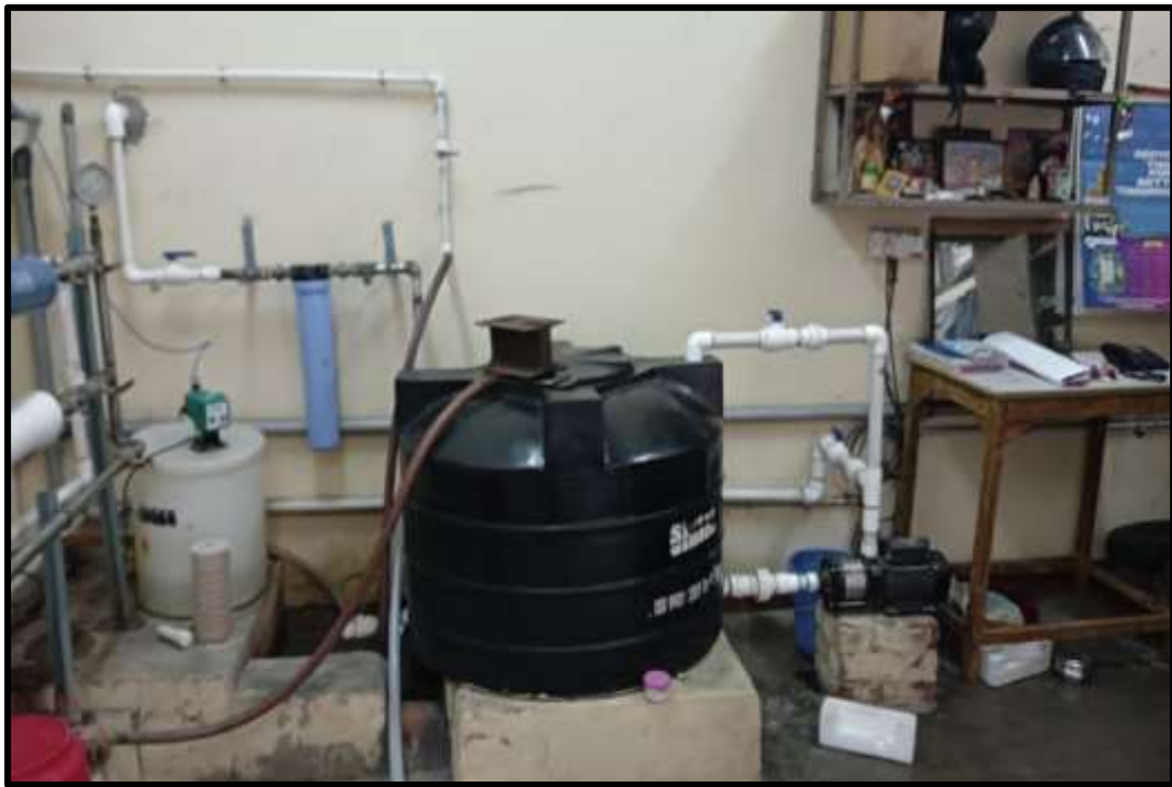
Water Treatment Plant Facilities
