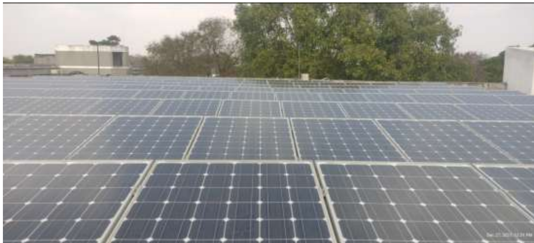
Solar panels installed above Academic Block
