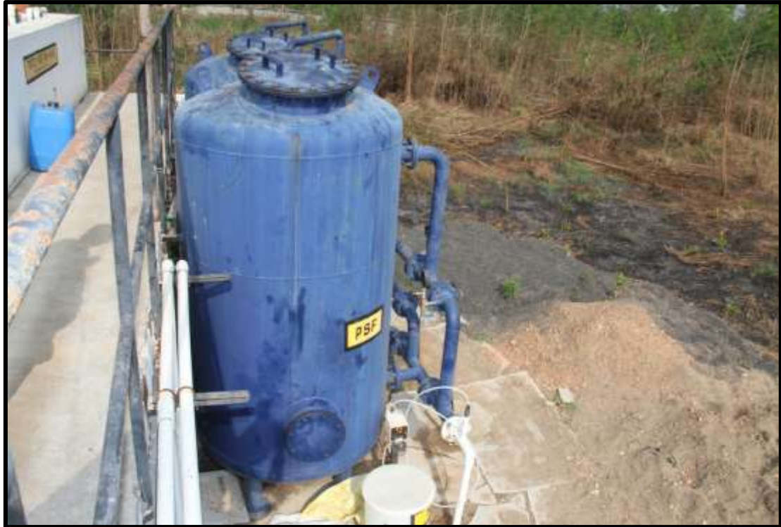
Pressure Sand Filter & Activated Carbon Filter
