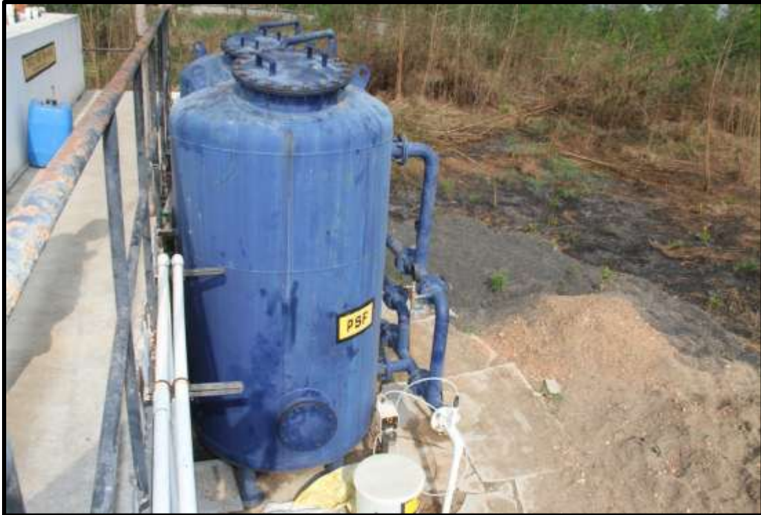
Pressure Sand Filter & Activated Carbon Filter
