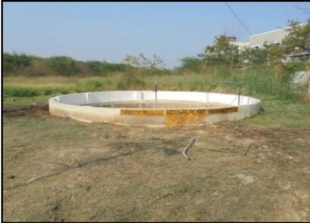
Bio Gas Plant
