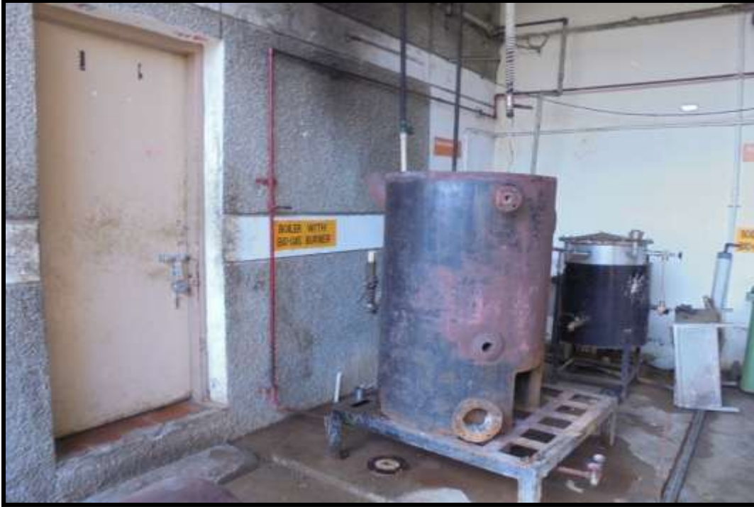
Boiler with Bio-Gas Burner
