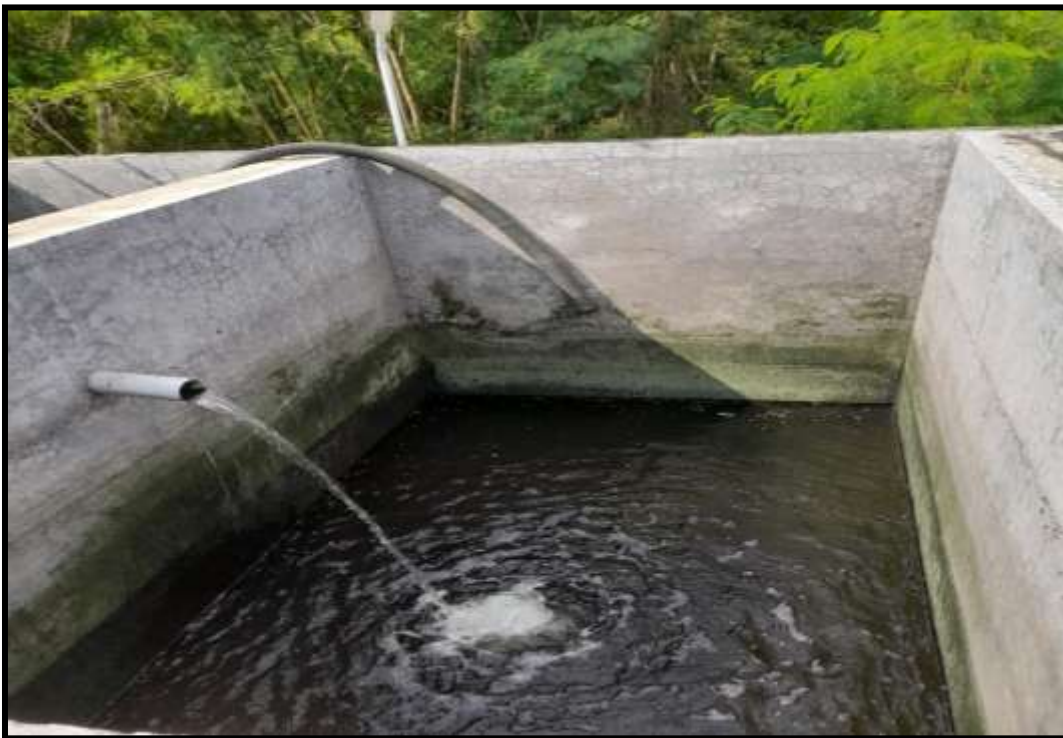
Clarified Water Storage Tank
