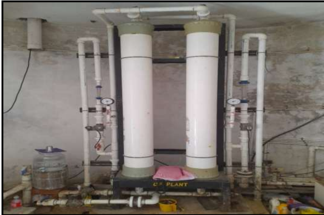
Ultra Filtration Plant
