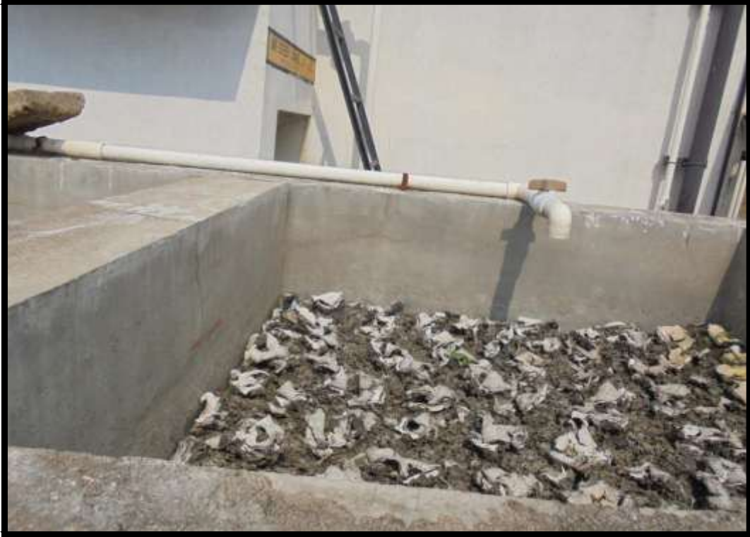
Sludge Drying Bed
