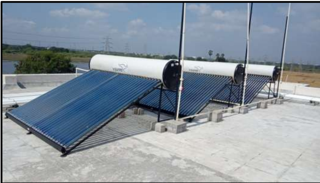
Photographs of Solar panels & Solar Water Heater
