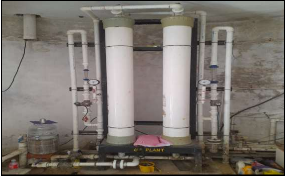
Ultra Filtration Plant
