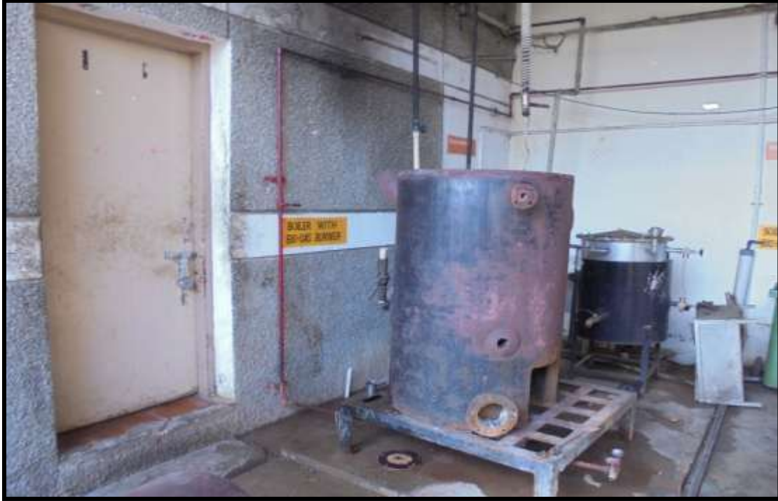
Boiler with Bio-Gas Burner
