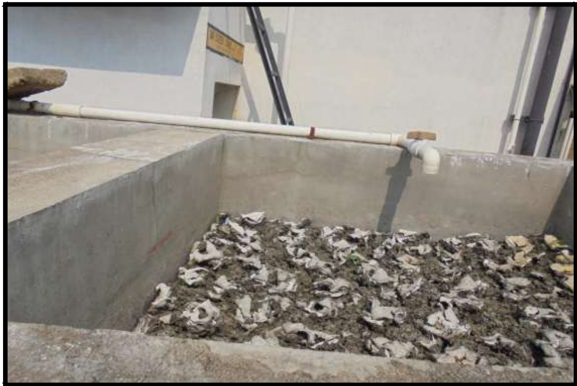
Sludge Drying Bed
