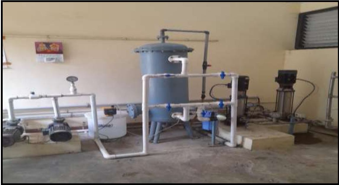
Water Treatment Plant – 200 KLD
