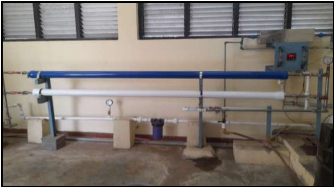
Sewage Treatment Plant – 250 KLD Capacities
