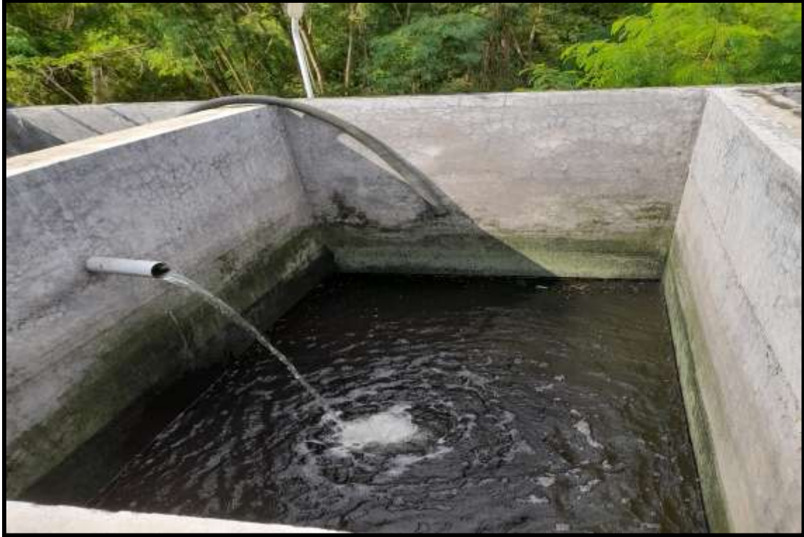
Clarified Water Storage Tank
