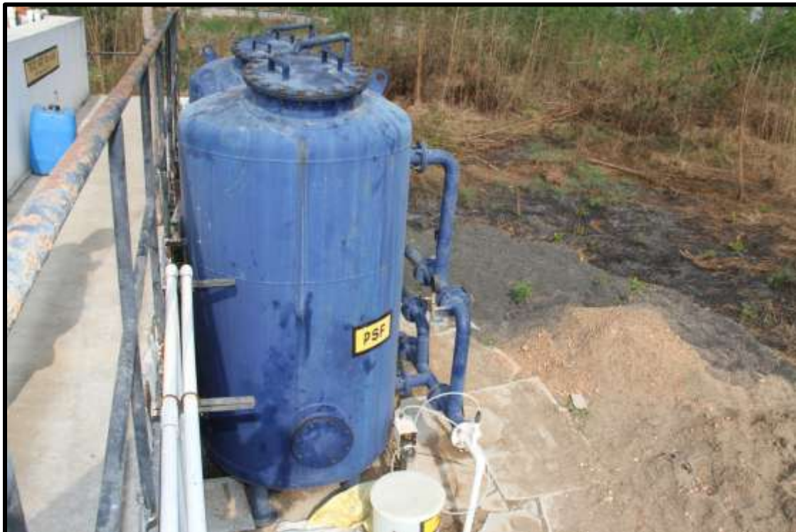
Pressure Sand Filter & Activated Carbon Filter
